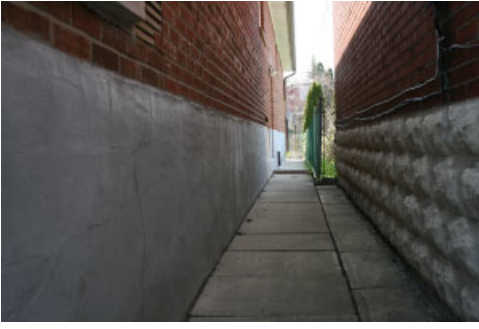
Walkway slopes towards foundation wall on west side of house.
