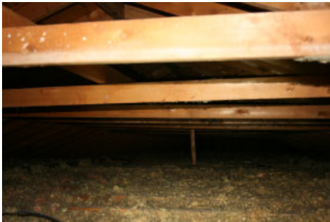
Low attic insulation
